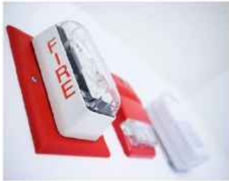
Visual Fire Alarms
