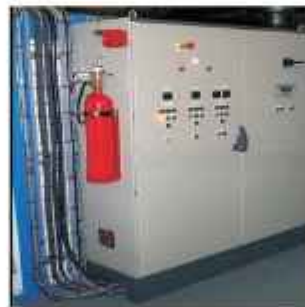
Figure: 4 CO 2 fire extinguishers, placed near major electrical panels (Picture Courtesy Wikipedia)
